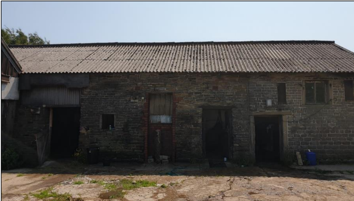
Plate 14 North-West elevation of 4 Greenside barn. The left hand side is the original 17 th century barn. The right hand side was added during the mid-late 18 th century
